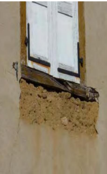
Water infiltration under the sill (SM)
