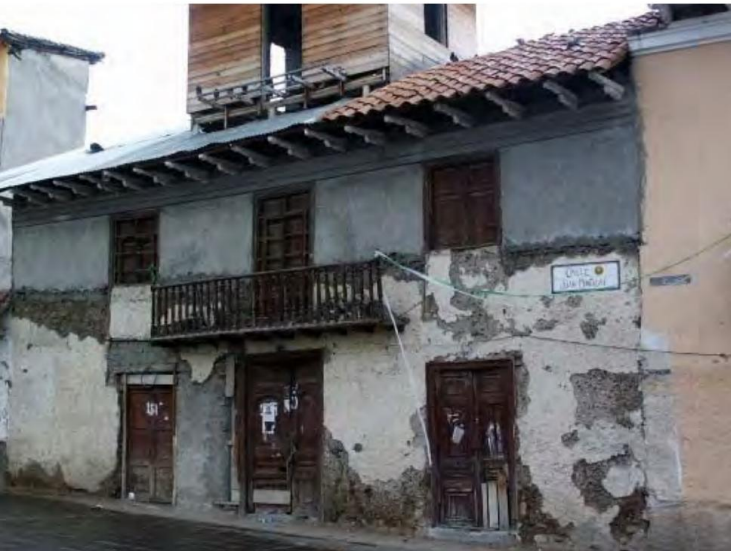
Adobe wall with detachment of the watertight plaster (LA)
