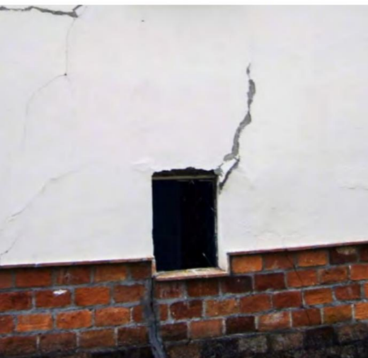
Little embedment of the lintels (LA)
