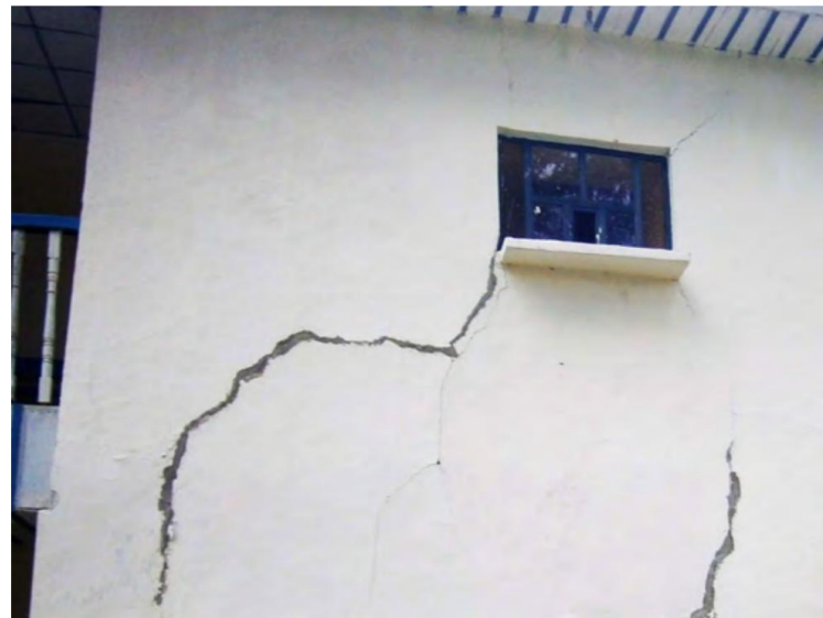
Foundation settlement cracks (upper crack) (LA)
