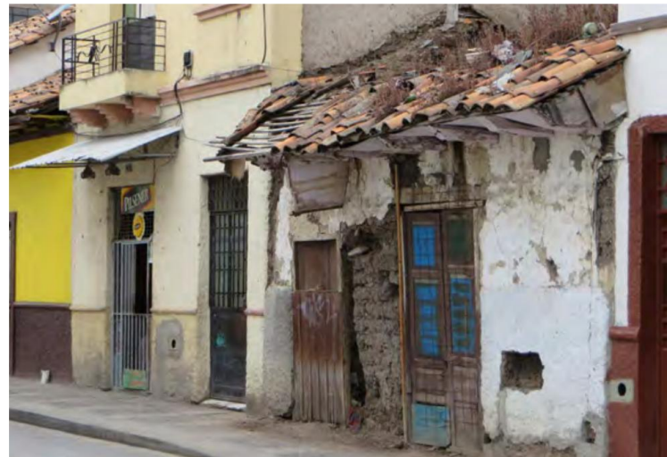
Ruined building in the Historic Center (ES)
