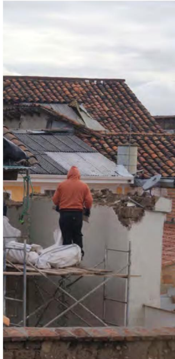
Adobe wall with dismantled collapse (lower image)
