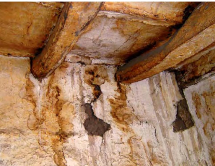
Water infiltration from the roof (DP)
