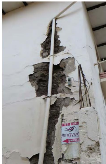
Defective downpipe (ES)
