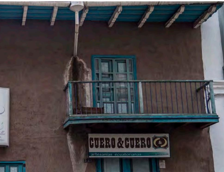
A faulty downpipe inside the wall is causing a water leak. (LA)
